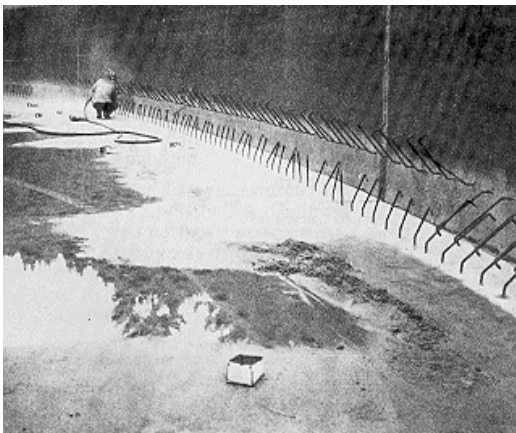
(Left) Reinforcement in the Chicago Park flume consists of 3/4-in. hookbars on 12-in. centers which were epoxy paste grouted.
