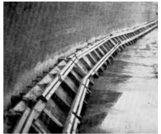
(Right) After sandblasting, wood forms were built. A very long potlife liquid epoxy bonding agent was sprayed onto concrete and steel, and a 6-1/2 sack portland cement concrete poured.
